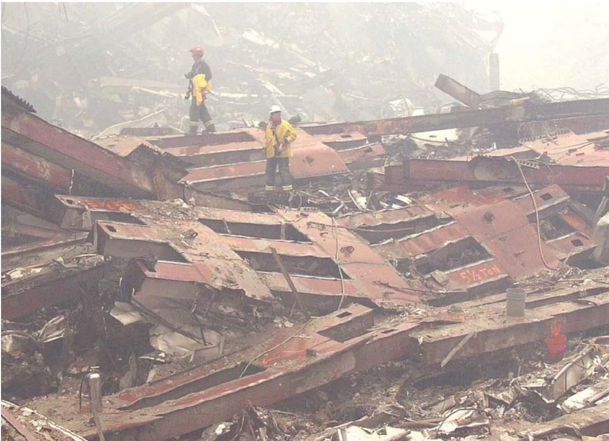
Figure 10 What caused these beams to wrinkle? We also note there is no "steam" rising from beneath these beams on a rainy day.
