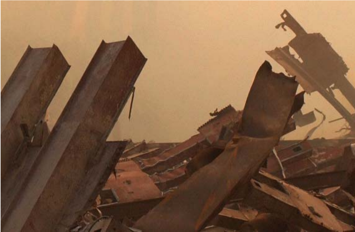
Figure 9 What caused these beams to wrinkle?
