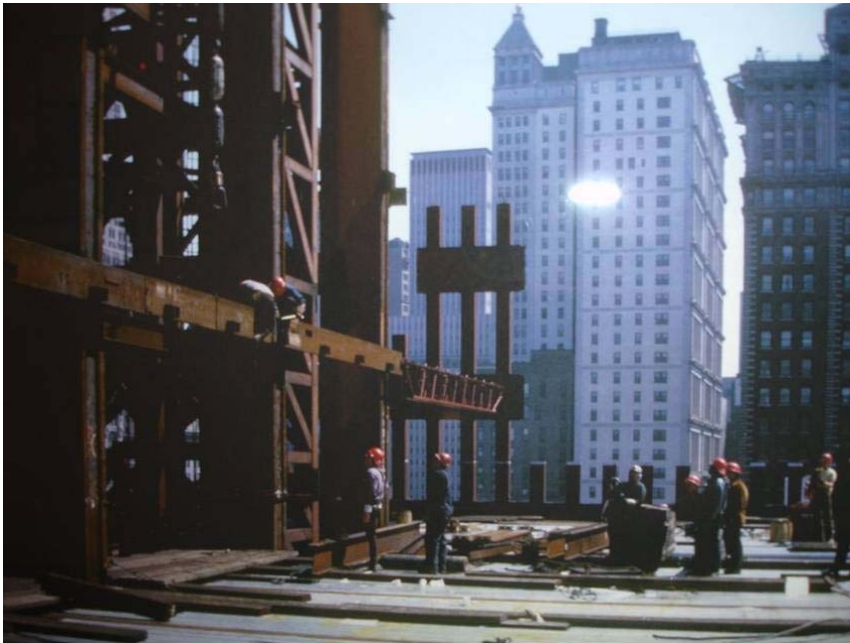
Steel-frame: Huge core (left) is an enormous heat sink. Notice workers standing on floor pan which is firmly attached to the interconnected core columns.
