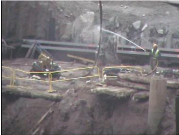
Figure 3 - Hosing down of a suspended cable at NYC WTC Site, 17th Jan 2008. Still image from Samsung MX10 Video Camera.
