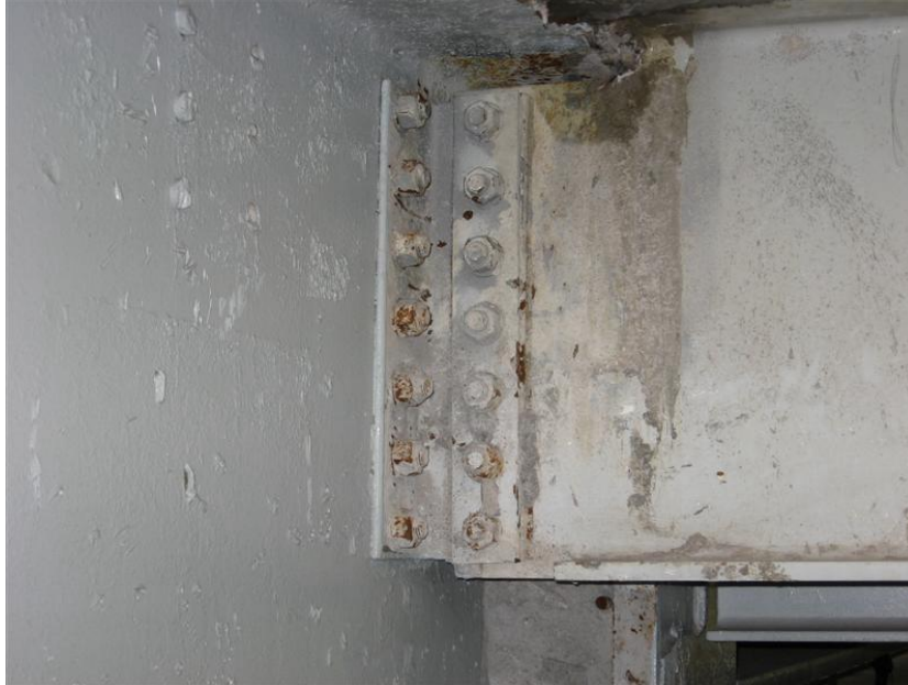
Figure 1 - Rusting/Corroded Beam on Path Train Station Stairway 17 th Jan 2008, Canon A540 Digital Camera
